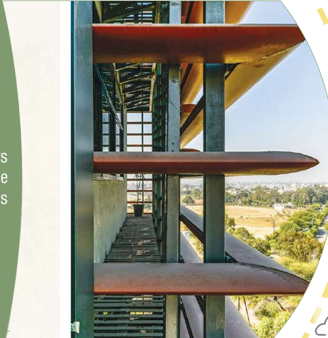
Close up image of horizontal louvers used installed at site to provide shading to the facade surfaces & reduce heat gain
