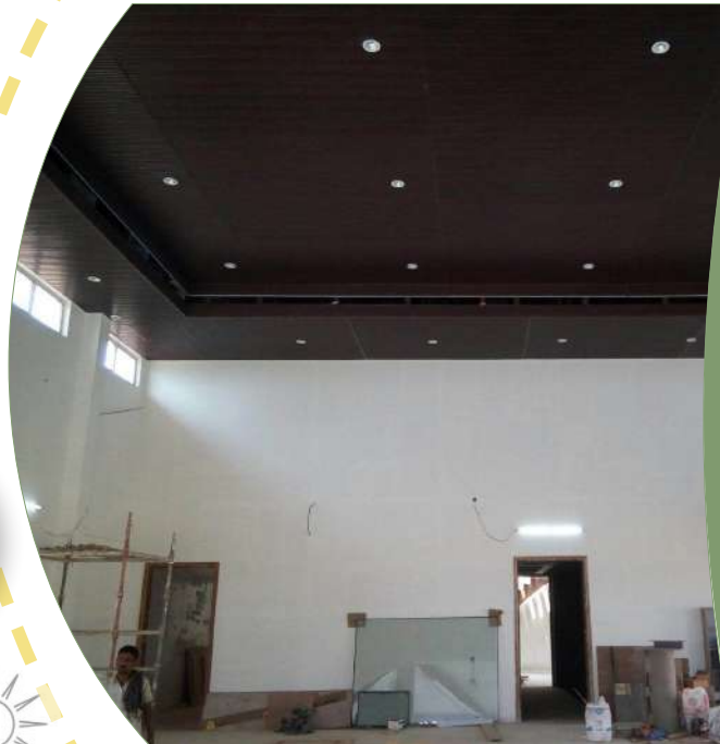
Image showing ventilators used for lighting & ventilation in double height space
