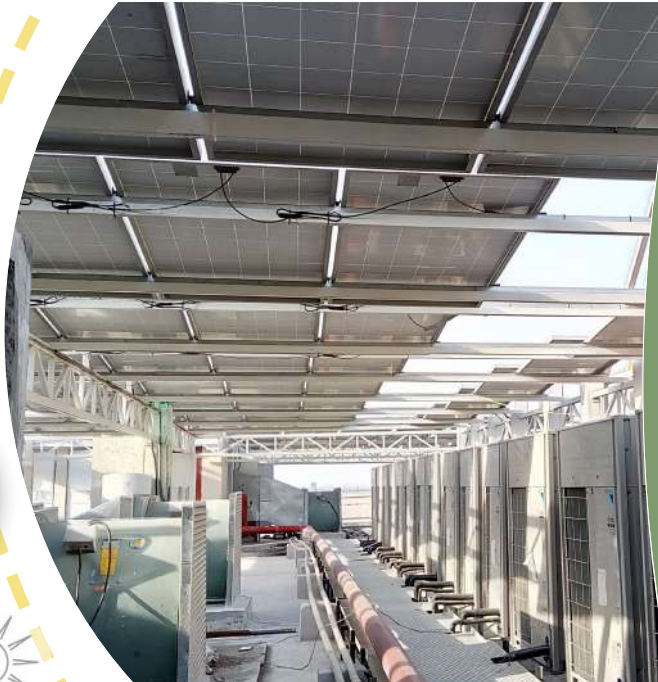
Image showing the solar panels on roof used to provide shade for service outlets & roof, reducing heat gain
