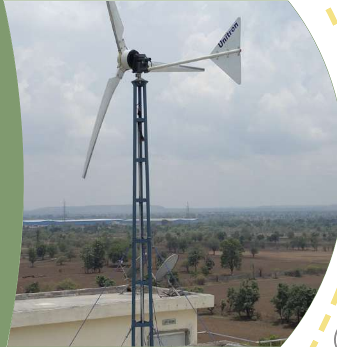
Image showing the wind turbine installed at the rooftop of the project for renewable energy generation
